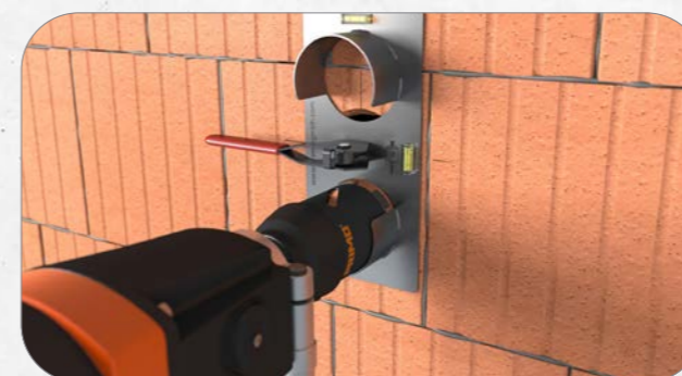
1. Mark the first box and drill out the hole using an 82 mm core bit. For multiple combinations, use the flush-mounting Drilling Template (P718).
